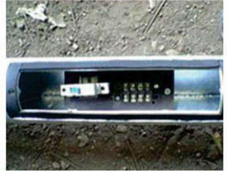
Inbuild Junction Boxes
