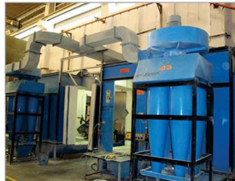
Powder Coating Booth, India Fully Automatic Conveyorized. Powder Coating Plant suitable for epoxy base Polyester Coating.
