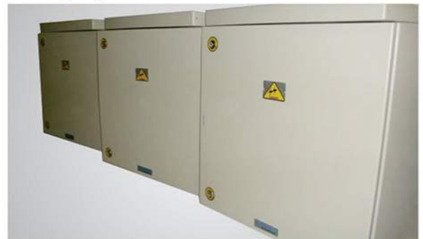
Outdoor Lighting Panel with Canopy
