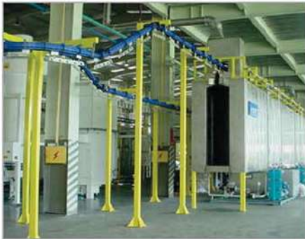
Conveyorized Surface Treatment (Make- Huali, China) Complete surface Treatment which involves processes like Predegreasing, Degreasing, Rinsing 1, DI Water Rinsing 1, NT 1, DI Water Rinsing 2, DI Water Rinsing 3, DI Water Spray.
