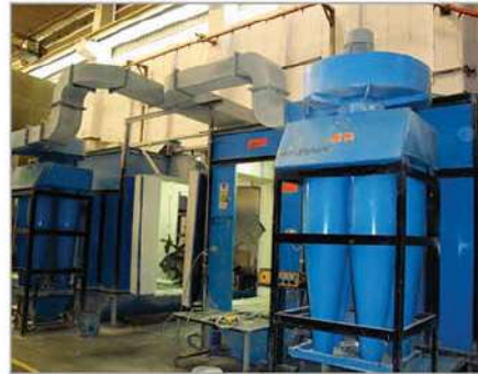
Powder Coating Booth, India Fully Automatic Conveyorized. Powder Coating Plant suitable for epoxy base Polyester Coating.
